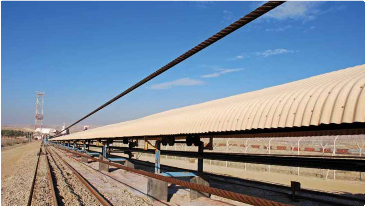
Project: Dead Sea Plant Conveyor - Israel | DURASHIELD® Type: White 1.5mm, Iron 76 Profile
